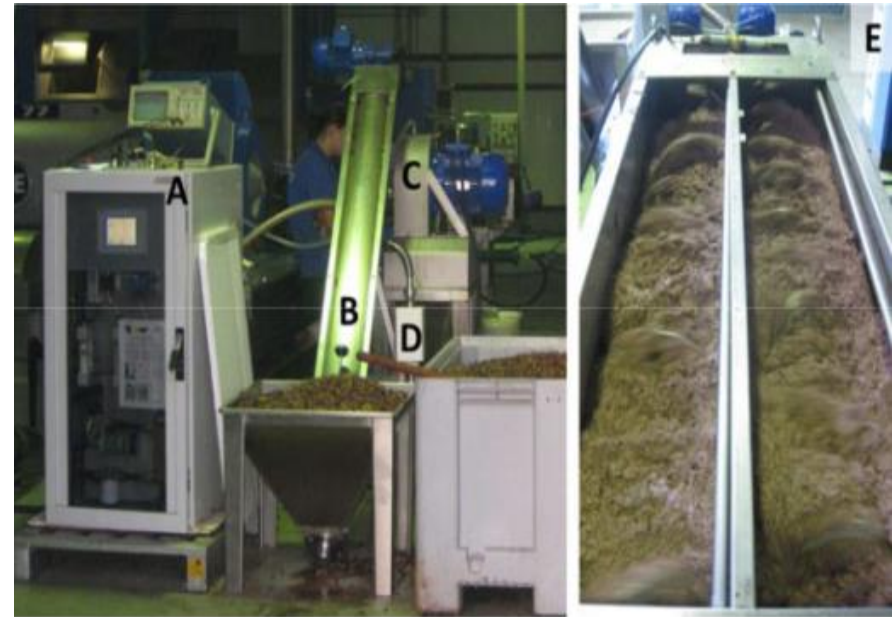
Setup for a pilot plant to study the PEF assisted recovery of olive oil. A) pulse generator; B) Crusher feed hopper and screw; C) Crusher; D) PEF treatment chamber; E) malaxer; F) decanter
